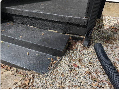
Foundation / stoop / steps - settlement (78-year-old house)
