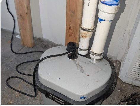
Two sumps + sewage ejector on GFCI
