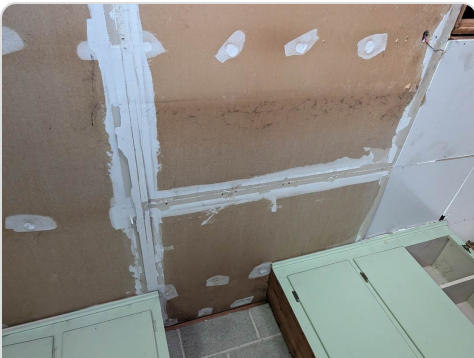
Garage - exposed wires + open junction boxes
