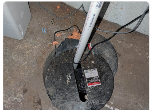
Sump lids open / askew
