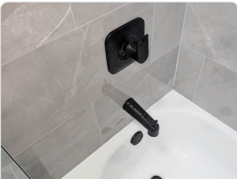
Shower valve installed incorrectly
