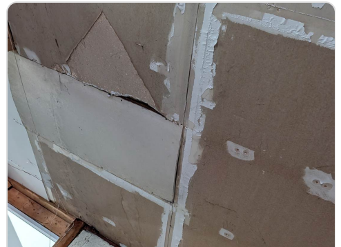
Garage ceiling - widespread finish / moisture damage
