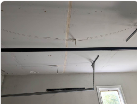
Garage ceiling - widespread finish / moisture damage
