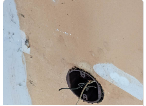
Garage - exposed wires + open junction boxes
